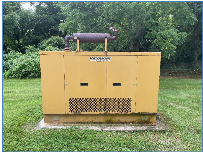
Figure 15. Photo of Water Tank Generator
