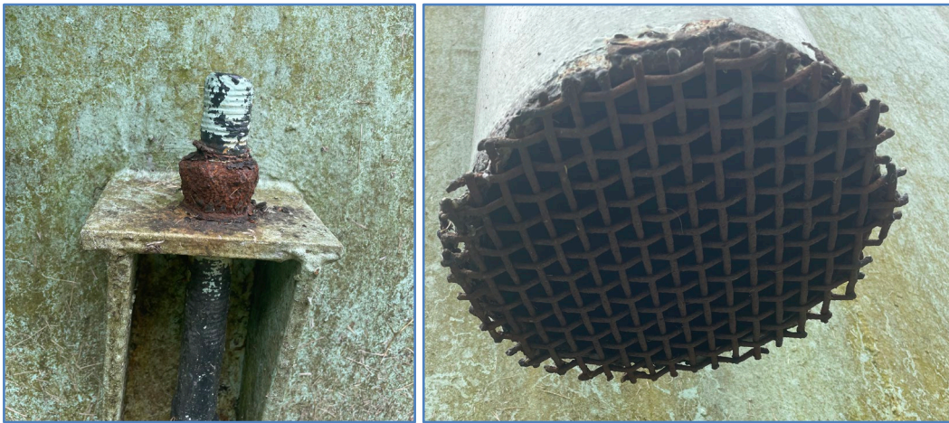
Figure 15. Corrosion on bolt (left) and overfill screen (right).
