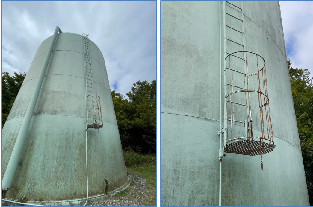
Figure 17. Ladder and ladder cage for water tank.
