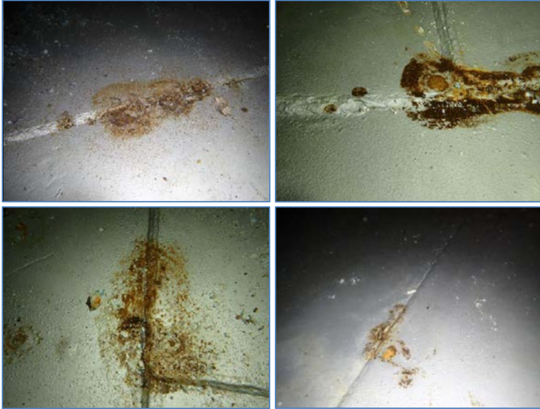
Figure 16. Corrosion on the internal welds of the water tank.
