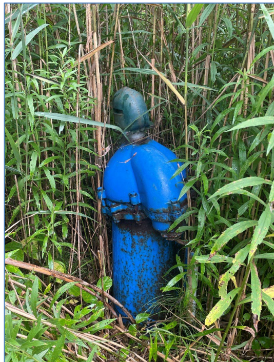
Figure 9. Photo of Well 4A
