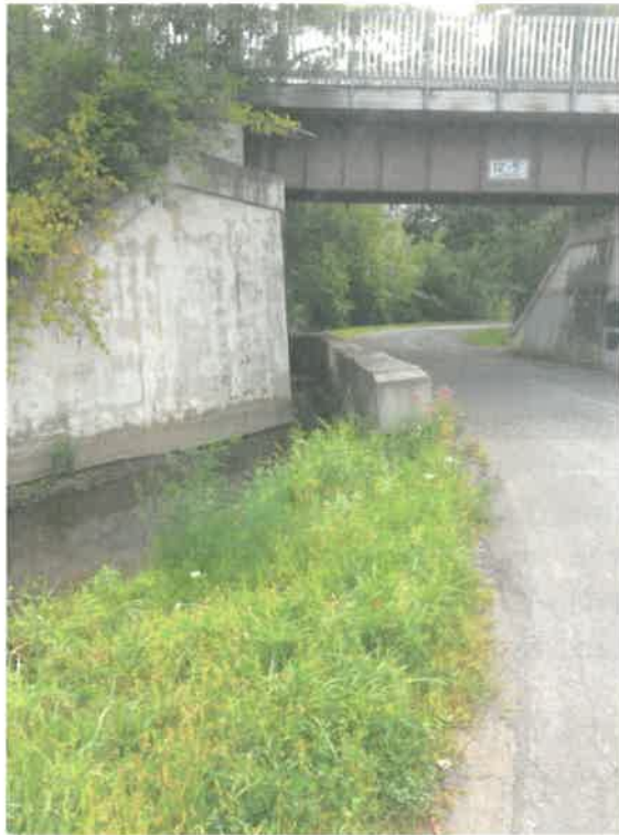
Above: Tributary channel being pinched between road and bridge abutment
