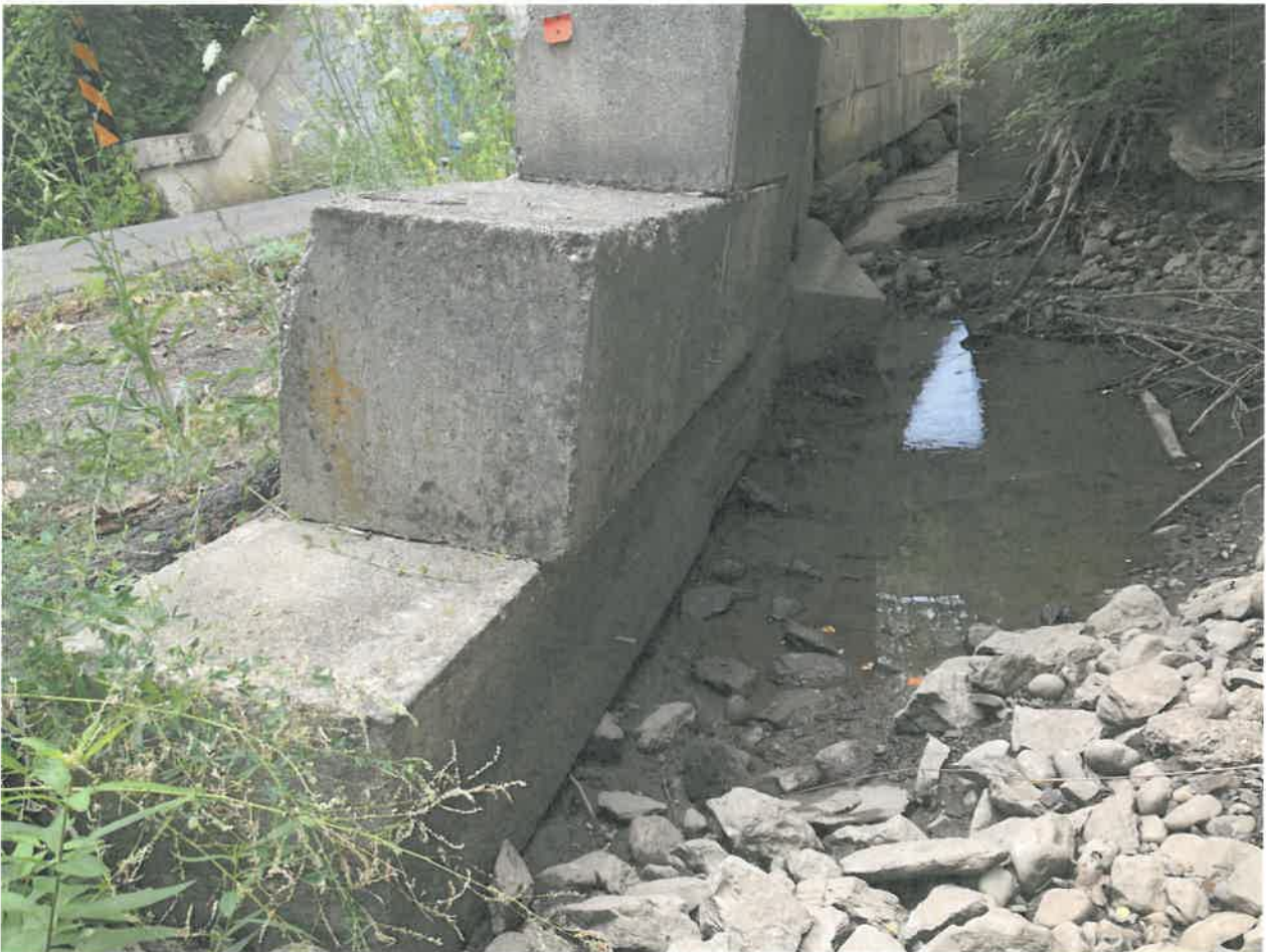
Below: Significant scour of structures and leaning concrete blocks
